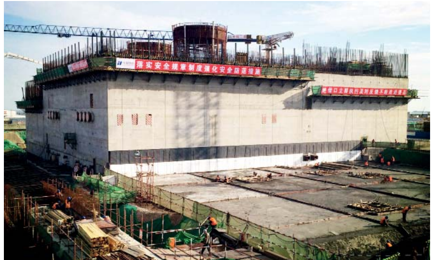
Fig. 13 – The construction of the Shidao Bay HTGR conventional island was finished on June 27, 2015 (photo credit: Shidao Bay NPP)
