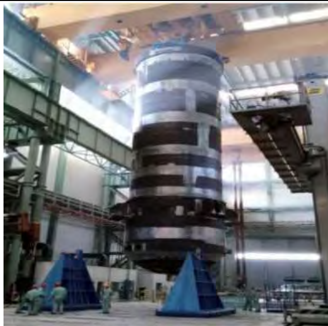
Fig. 4. Manufacture of the HTR-PM reactor pressure vessels by the Shanghai Electric Corporation; status as of September 2015. (Bild ist optisch verzerrt )
